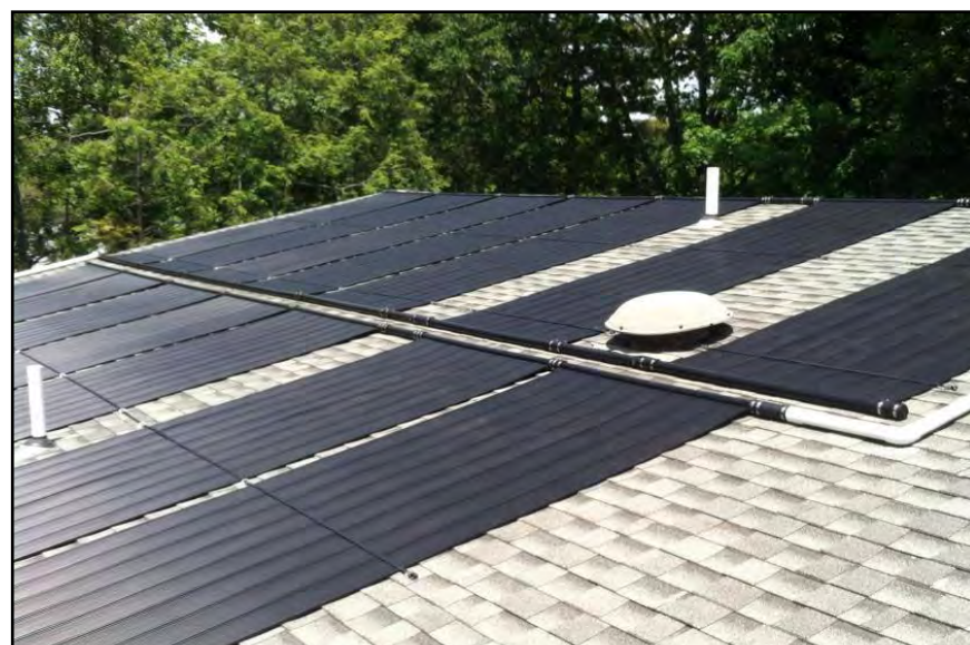
Using various configurations of hoses and header spacers, this system avoids roof obstructions while maximizing the solar collector area. (Photo courtesy of Solar Living - Fair Lawn, NJ)
